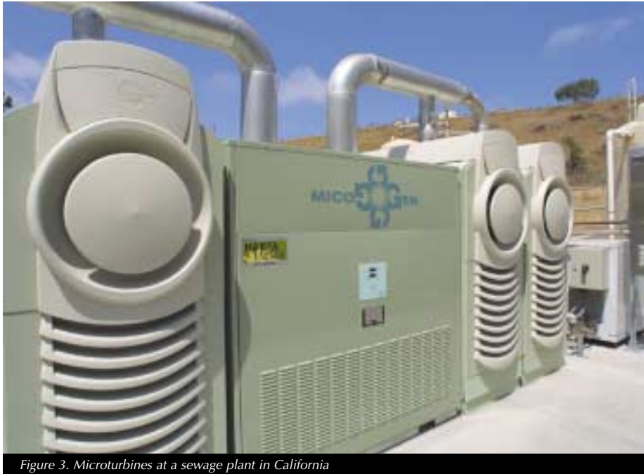
Figure 3. Microturbines at a sewage plant in California
