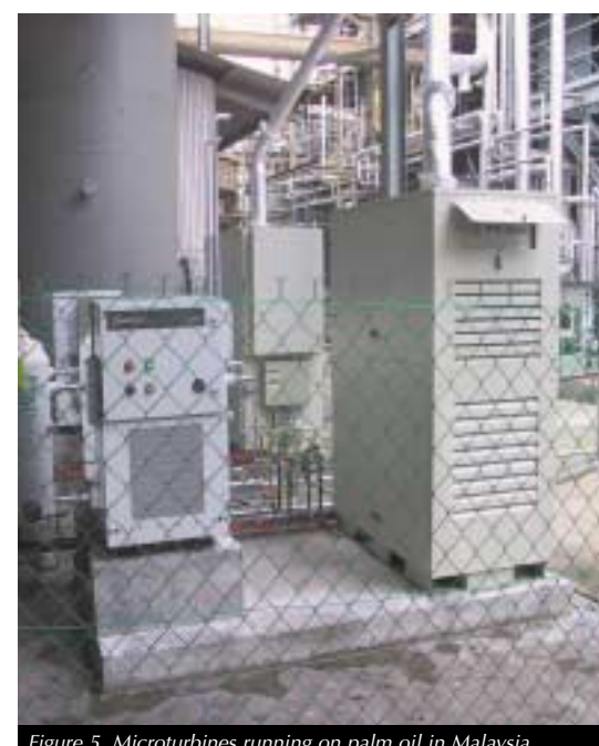
Figure 5. Microturbines running on palm oil in Malaysia
