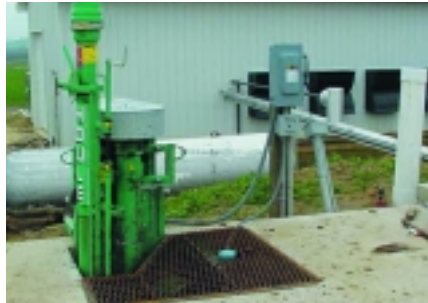
The slurry pump (foreground) and the cogeneration room (background) at one of Alliant Energy's farm-based digester/cogeneration projects
